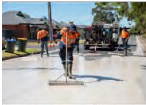
Figure 4: Coolseal finish applied to roads in City of Charles Sturt to reduce the urban heat island affect.
