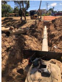
Local Flooding Trenerry Avenue Ingle Farm
