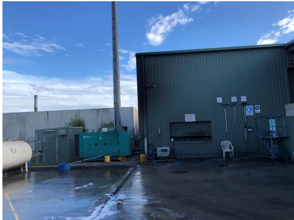
Photo 4. Looking north west from the hardstand toward existing site generator, mobile phone tower is in the south-western rear corner of the site
