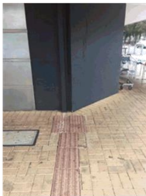
Figure 4-7 Incorrectly installed tactile markers
