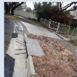
The Local Flooding Program delivered a variety of engineering solutions across the City
