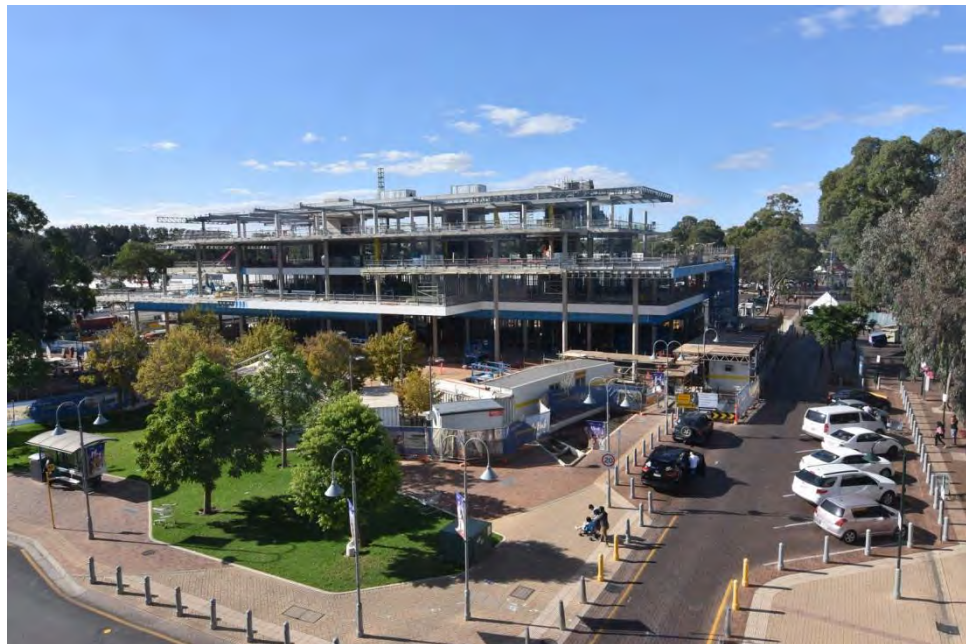
Photo 2: Roof Plant Slab upstands complete, Steel Roof Structure complete, Formwork stripping complete (Photo: 22 April 2019)
