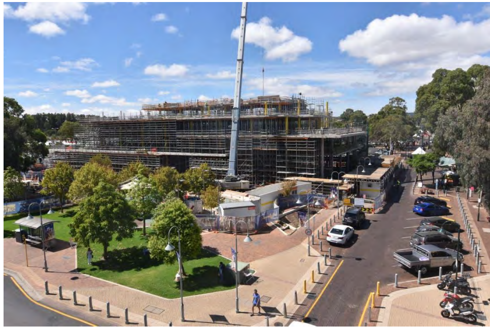
Photo 1: Roof Plant Slab complete, Steel Roof Structure Installation, formwork stripping commenced on John Street (Photo: 21 January 2019)
