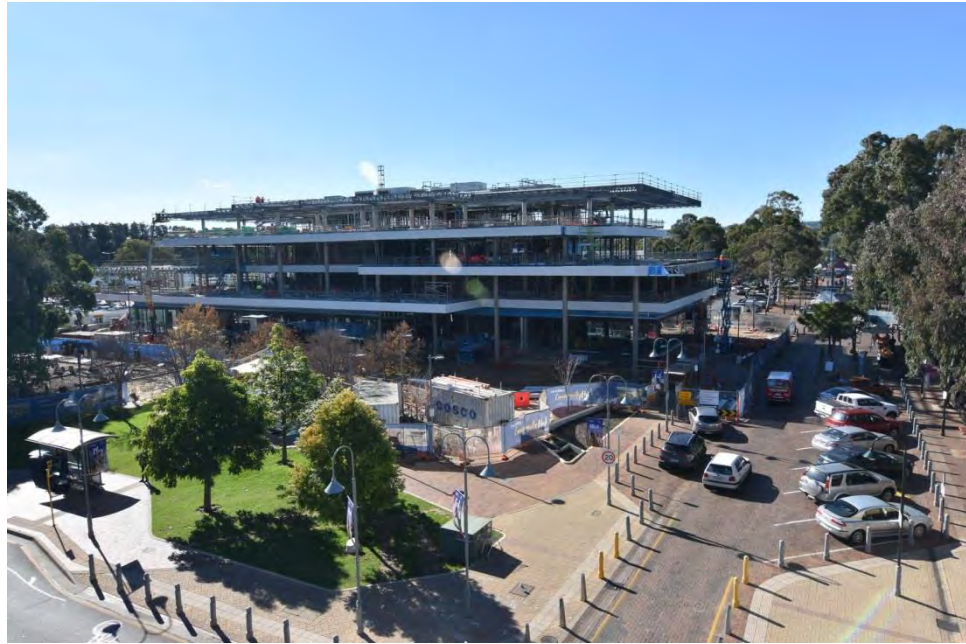
Photo 3: Roof Plant Slab upstands complete, Steel Roof Structure complete, Formwork stripping complete, Slab Edge fascia cladding and Ground Floor Glazing (Photo: 7 June 2019)
