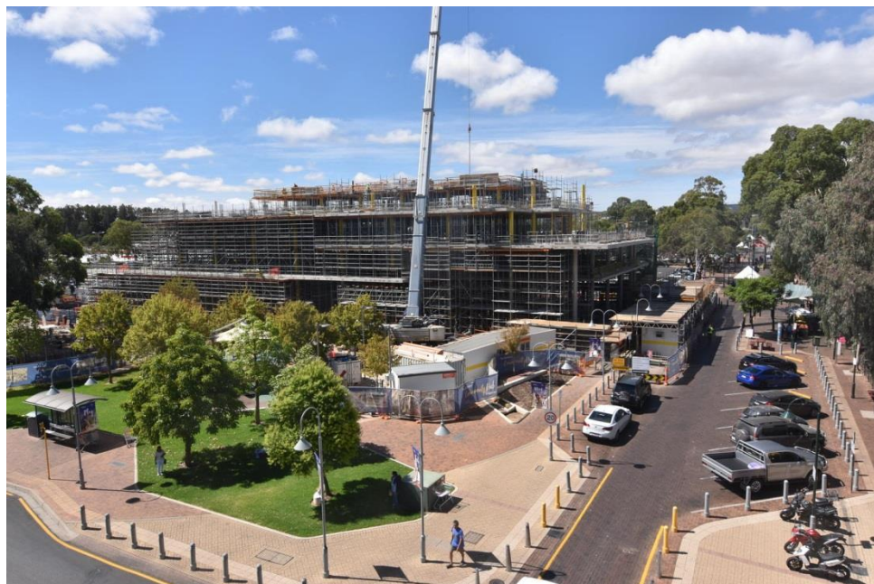
Photo 3: Roof Plant Slab complete, Steel Roof Structure Installation, formwork stripping commenced on John Street (Photo: 21 January 2019)
