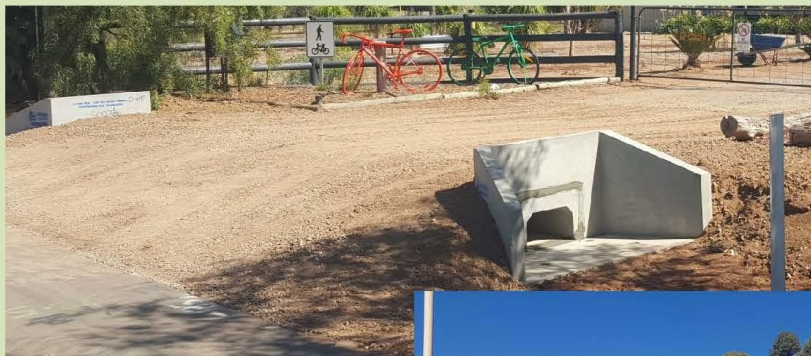
Local Flooding Program Barker Road, St Kilda
