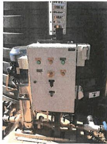
Wastewater manifold and discharge pump
