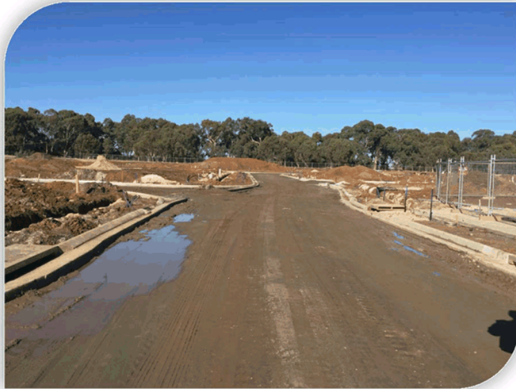
Photo 2 - Boardwalk Drive under construction, Council's fifth residential housing development delivering 122 residential allotments.
