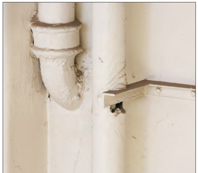
Damaged and exposed pipe wrapped with asbestos lagging
