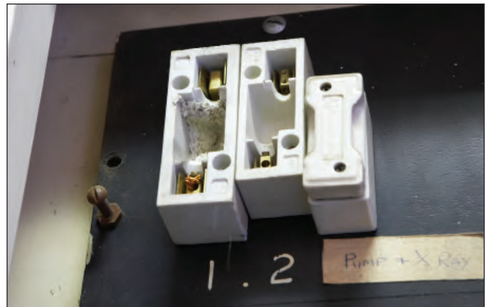
Friable asbestos insulation in an electrical fuse housing
