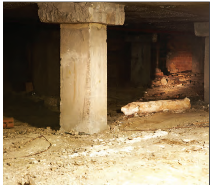
Unfixed asbestos lagging from a pipe
