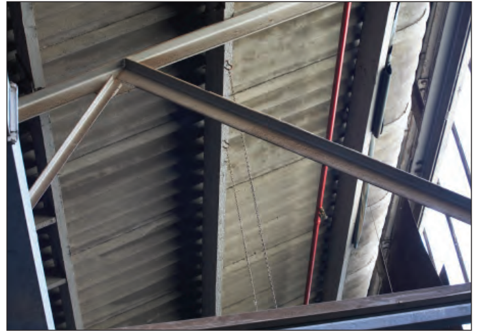
Underside of asbestos cement roof cladding.
