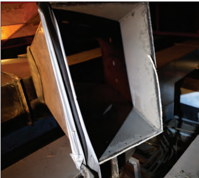
Detached asbestos rope seal and remnant debris on duct.
