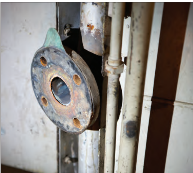
Asbestos containing gasket
