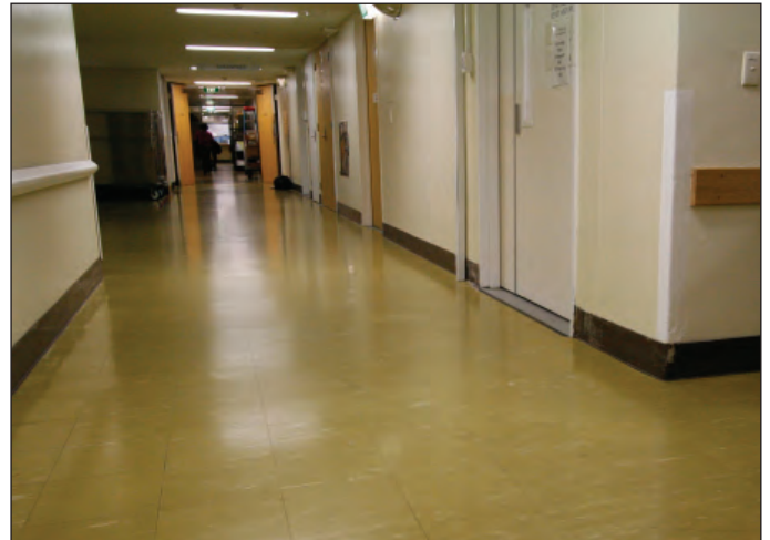
Asbestos vinyl tiles
