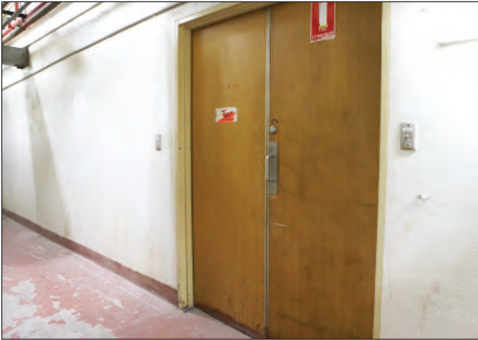
Fire rated door containing asbestos
