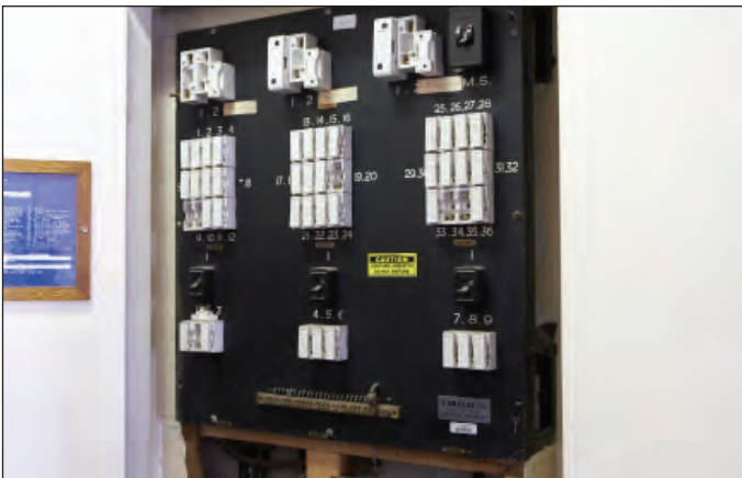
Asbestos containing zelemite electrical switchboard panel
