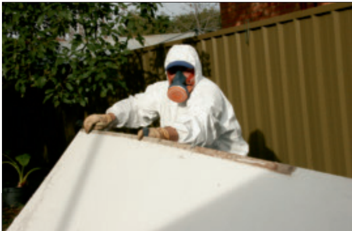
FULLY LICENSED ASBESTOS CONTRACTOR REMOVING THE ASBESTOS-CONTAINING UNDERLAY TO VINYL SHEET FLOORS.
